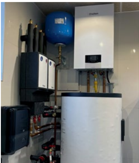
Kotlovnica restorana Avangard
